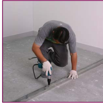
2. Attach U76 on the floor, ceiling and aside of the wall follow the mark using concrete bolt in every 30 cm.
